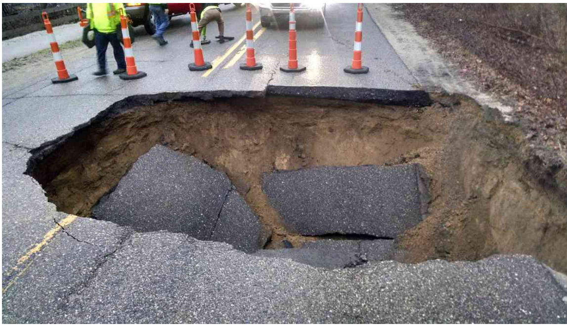
Figure 7. Collapsed section of 148th Avenue in Spring Lake Township after a culvert failure. Image from Grand Haven Tribune online article (link no longer available).
