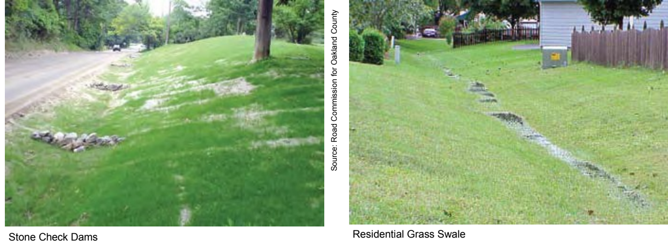
Stone Check Dams Residential Grass Swale
