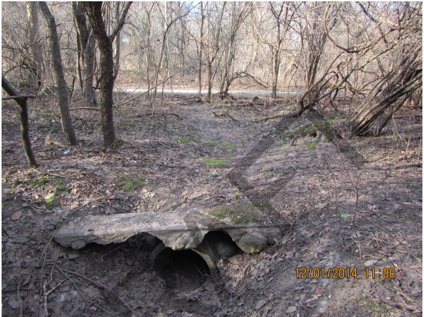
Photograph 5: Richards Fairplains Drain Outfall in Huff Park
