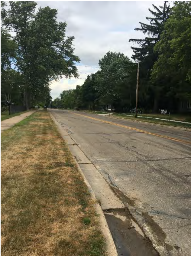
Awixa/Richmond on 7-20-18. All soak up was swept up. Some staining remained in gutter.
