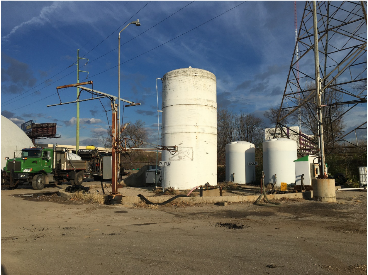
Calcium Chloride tank and secondary containment.
