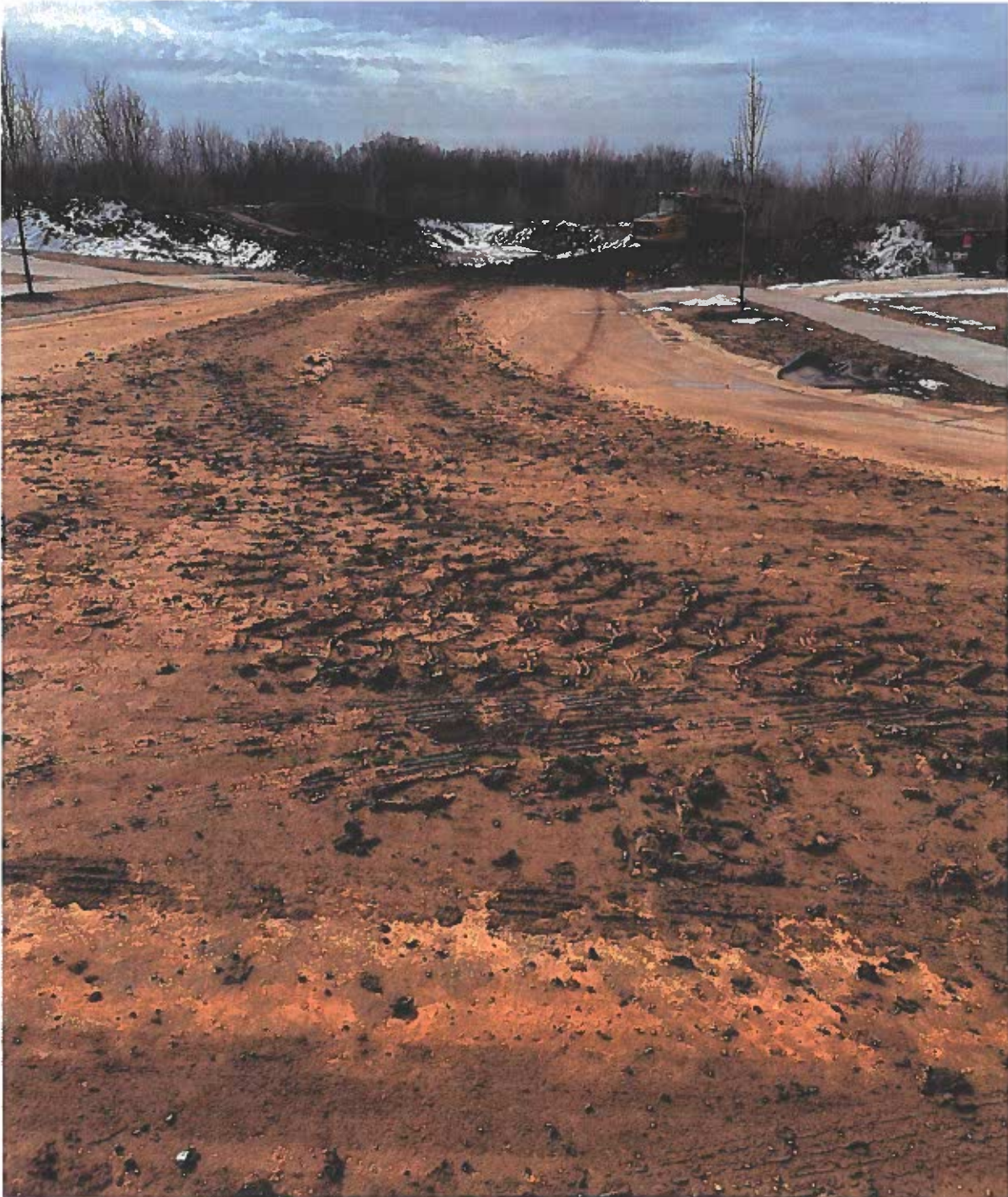
Picture 1. Tracking due to lack of controls at construction entrances. Stone needs to be installed and maintained to help eliminate tracking.
