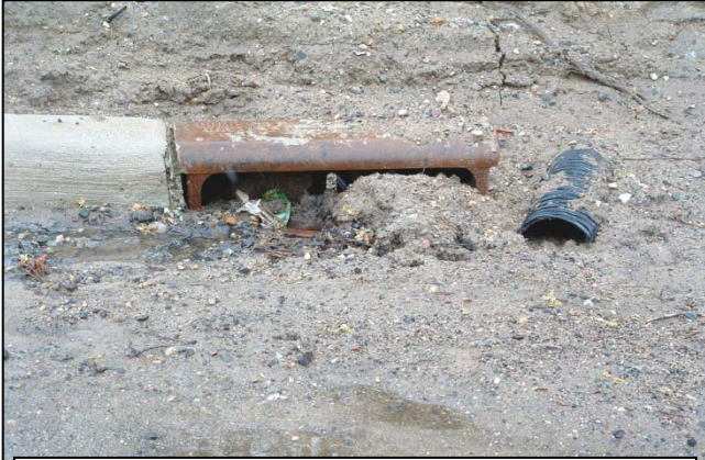
Excessive sediment from construction site.
